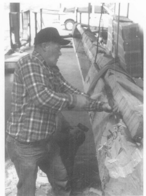
Figure 6. Three of the 7 totems had support posts. The steel bolts connecting the support posts to the totem had rusted and often needed to be chiseled out of the support post. Note the hollowed back of the totem which extended nearly the entire length while the support post extended only about half way.
